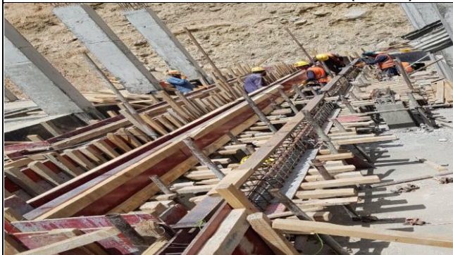
Formwork installation and steel fixing of indoor cable trenches at grid station.
