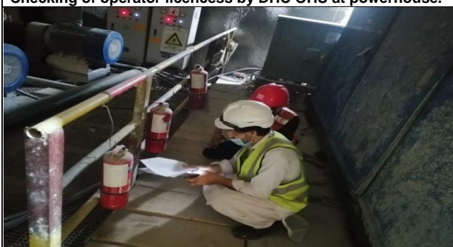
Monthly inspection of CGGC fire extinguisher inside the tunnel
