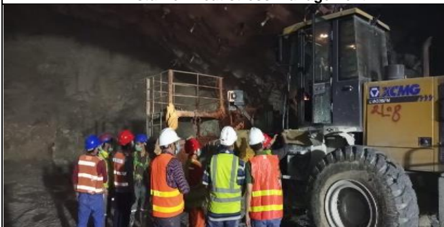
Checking of operator licencess by DHC OHS at powerhouse.
