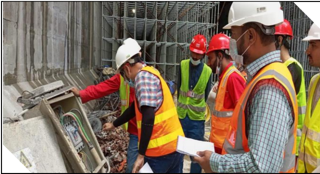
Electrical DBs inspection at DTA Inlet by DHC OHS
