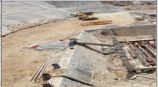
Clearance of Upper Terrace for installation of electrical equipment in Grid Station.
