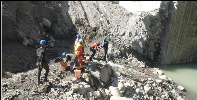
DT-A Inlet Date 14-04-2023
