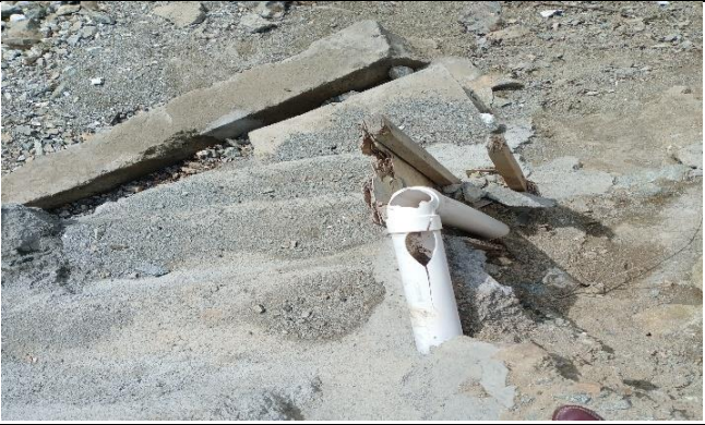
The broken internal water supply pipeline at Rv Uchar-01
