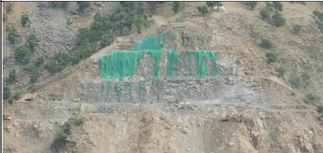
Right Bank Cable Crane Date 18-04-2023
