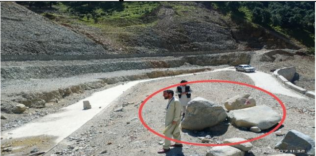
The encircled point is the area where Septic tank is constructed underground at RV Khushi-02 Link-01
