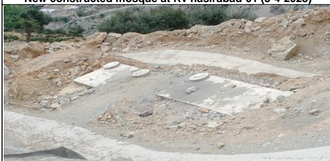
Septic and anearobic tank at RV Nasirabad-02
