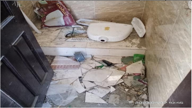
The broken flushing tank in the toilet at RV Khushi-01
