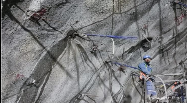
PH. 79-2 PS tendon washed by contractor..
