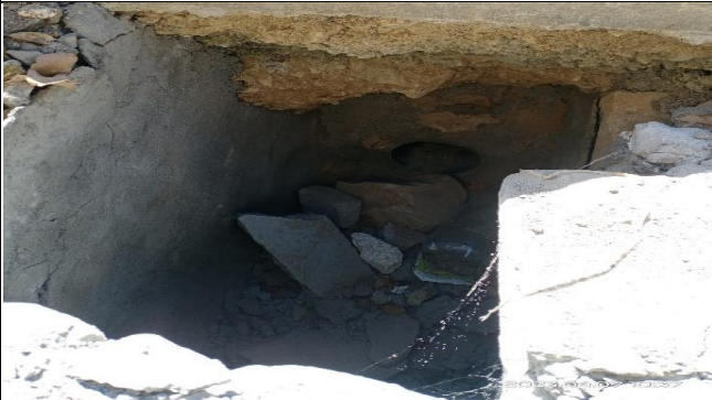
The broken manholes of Swerage line at RV Khushi-01
