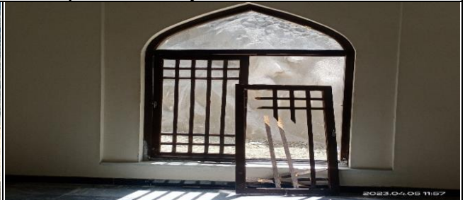
The broken window of Mosoque at Rv Nasirabad-01 (5-4-2023)
