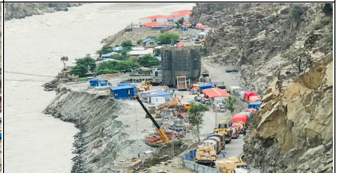
MW01- Facilities for DTs at CR2
