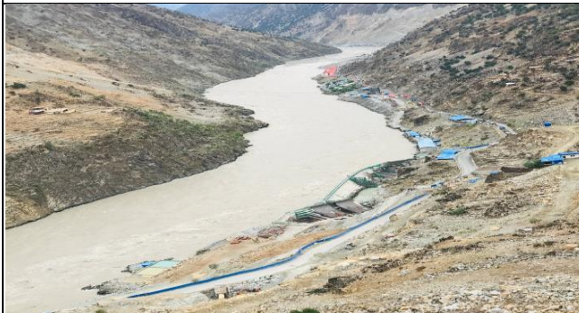
MW01- Facilities for DTs at CR2
