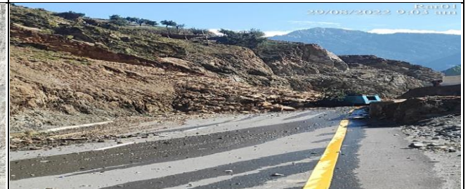
Slided Material around K11+500 area (RAR-01)
