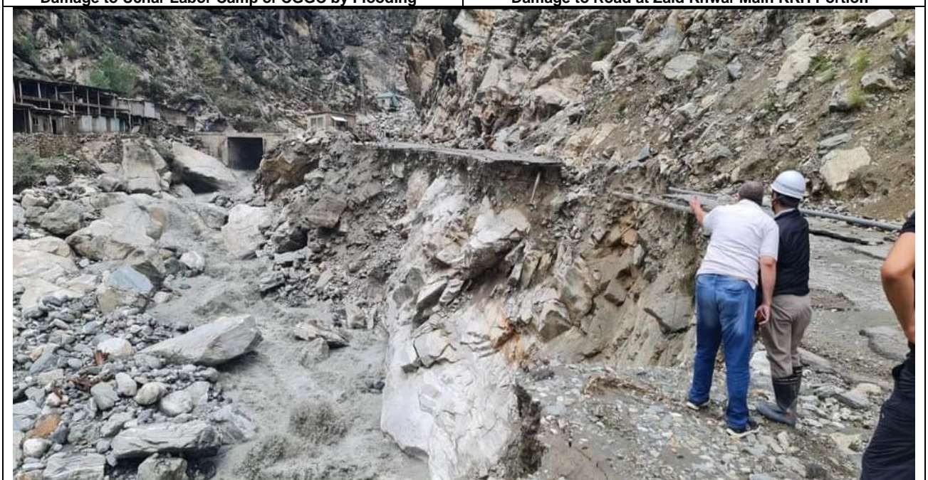
After Road Washed Away at Zaid Khwar Nullah on 28th of Aug 2022
