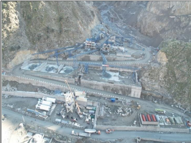
Uchar Thoki – Crushing Plant & Batching Plant (MW-01 & 02)
