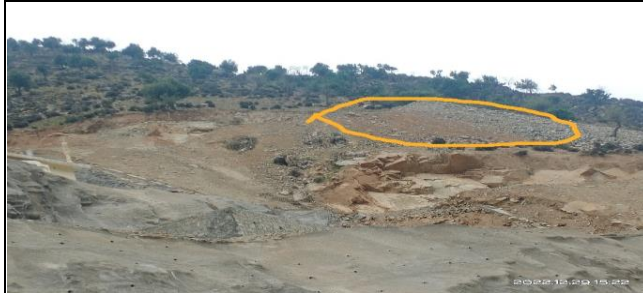
Contractor had not removed the encircled disposed excavated Loose Materials from the corner of middle terrace at RV Nasirabad-01
