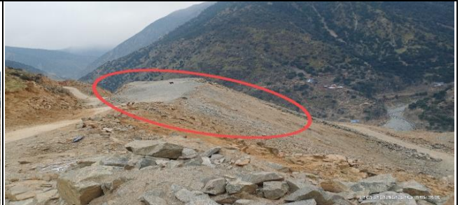
Resettling villagers also demanding the contractor to remove the encircled loose materials dumped at the entrance of first terrace at RV Nasirabad.
