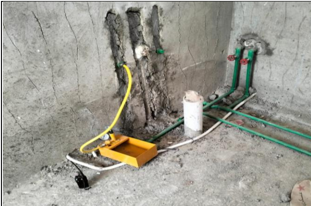
PPR Testing at Cat 2
