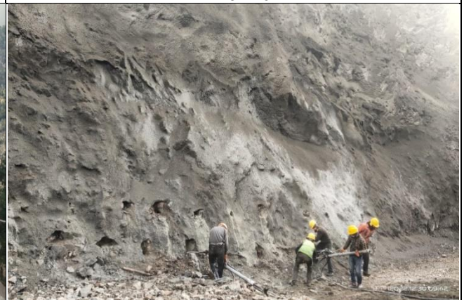
Drilling for rock bolts at Dugah Tunnel outlet Area for slope protection
