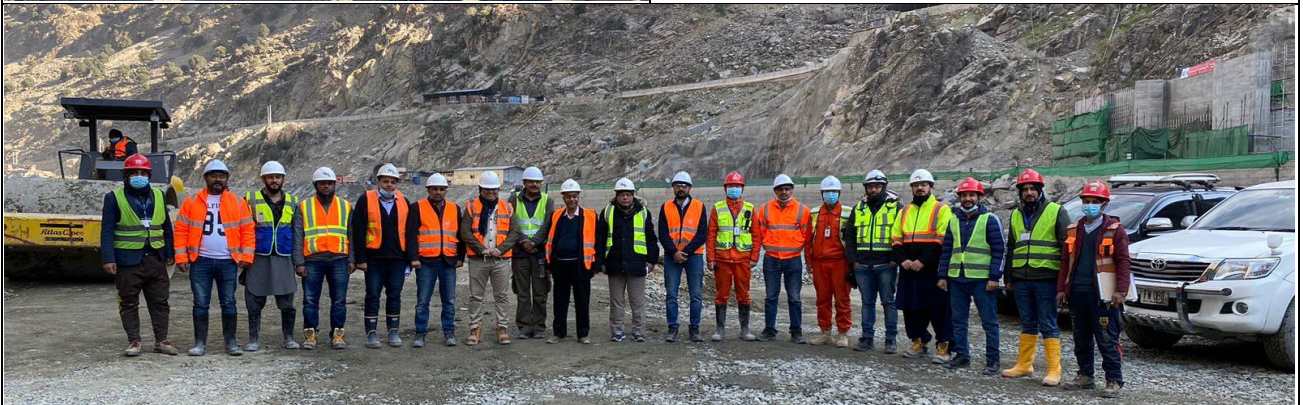
WB Visit to DHP K-09 Tunnel and Cofferdam Site on 22 nd of Dec 2022
