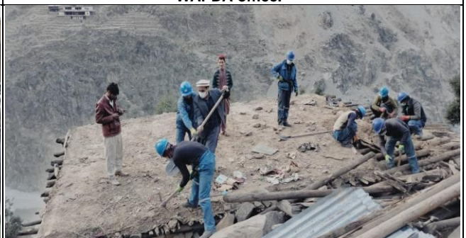
Demolishing of SMR Paid Houses by the Taskforce in the Project Area.
