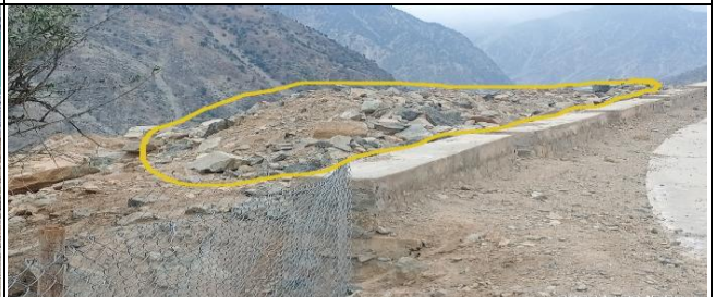
Contractor had not removed the disposed excavated Loose materials from the outer edges of Access Road at RV nasirabad-01
