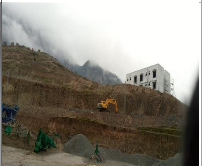
Excavation of water supply & sewage line at S 5 Road For Hostel cat 2B & 2A
