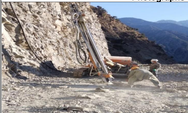
Right bank cable crane platform
