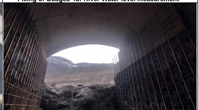
DT-A outlet inside
