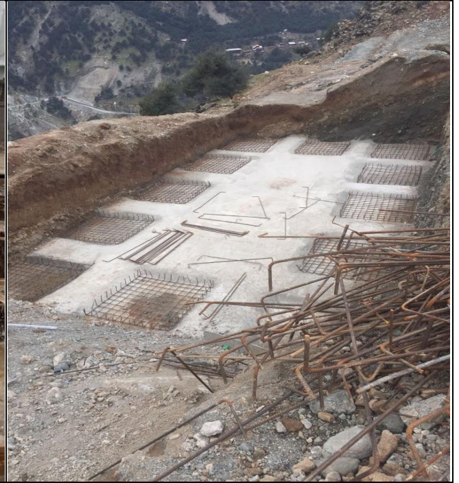
Main Septic tank Type A near relocated KKH steel fixing is in progress
