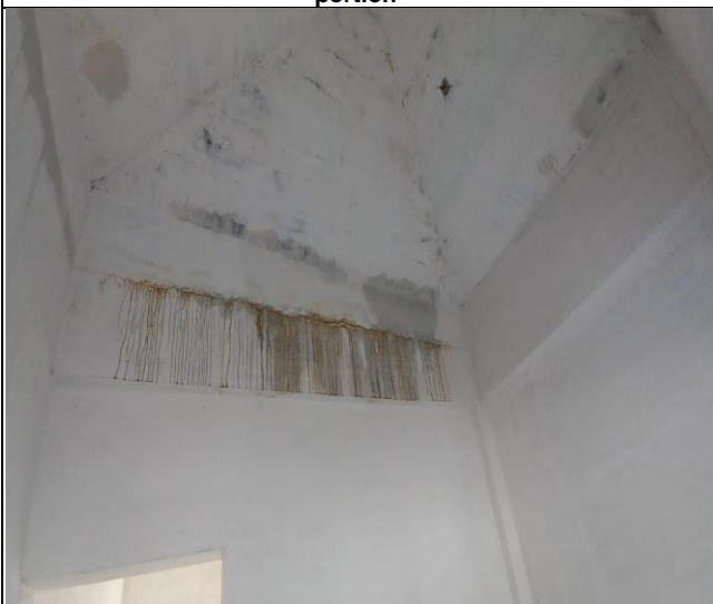
Cat 2B part 12 seepage at Dome
