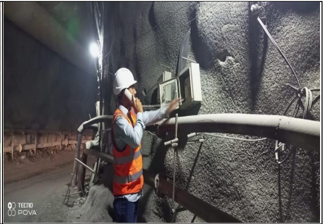
Checking effectiveness of communication system at STC junction by DHC OHS
