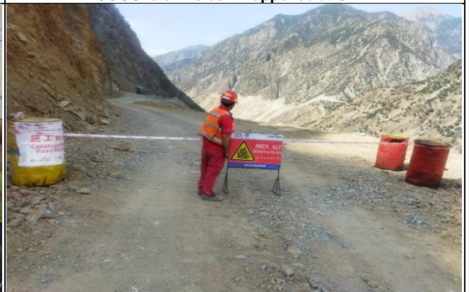
A view of road closure and signage during blasting operation at RAR-02
