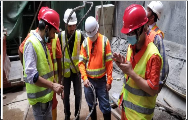
Inspection of sling/rigging equipment carried out by DHC OHS during joint inspection of tripartite at DTA
