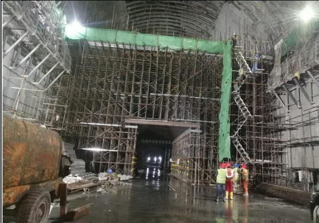
MW-01_ Fixing Formwork for concrete at Shear zone of Diversion tunnel B
