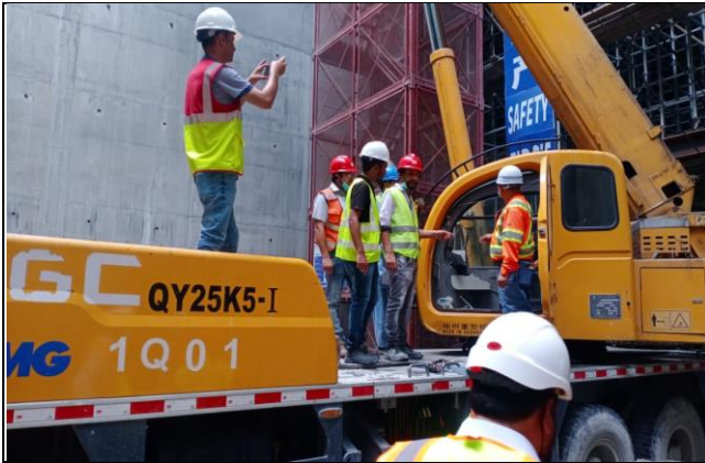
Inspection of crane carried out by DHC OHS during joint inspection of tripartite at DTA
