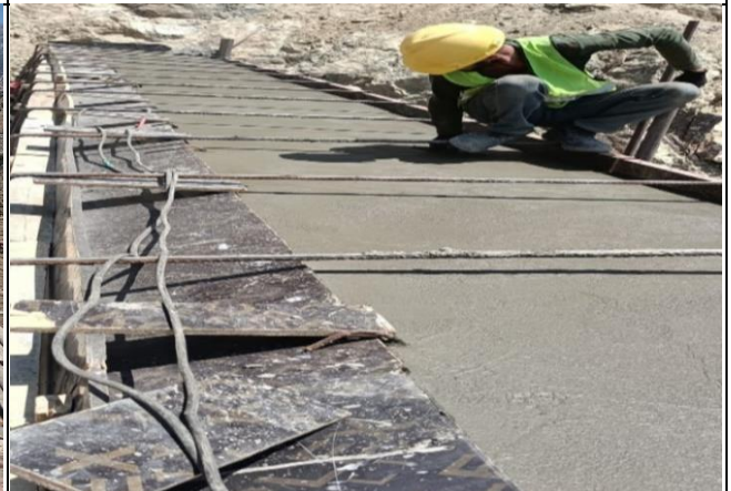
Concrete pouring of Sismic reinforcement wal completed at outlet of K3 Tunnel
