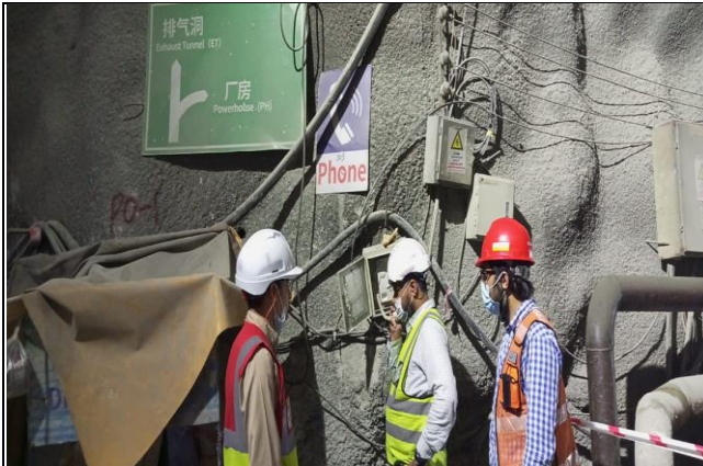
Checking effectiveness of communication system at powerhouse junction during joint inspection of tripartite at power house
