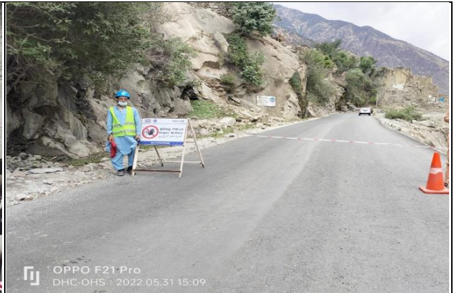
A view of road closure along with flagman and signage during critical activity at KKH-02
