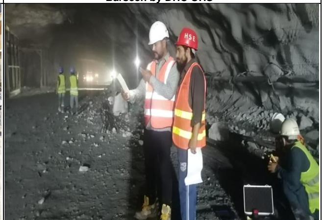
Validation of Air quality monitoring inside the tunnel by DHC and CGGC OHS staff
