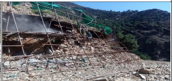
24-06-2022 Right bank cable crane
