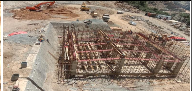
Formwork installation and steel fixing for top beam and roof slab concrete
