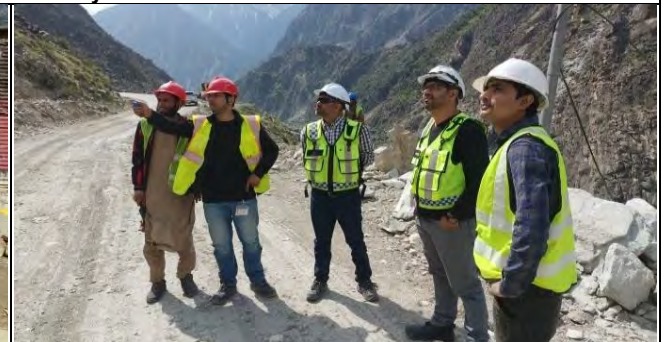
A view of joint inspection conducted with WAPDA, DHC and CGGC at KKH-02
