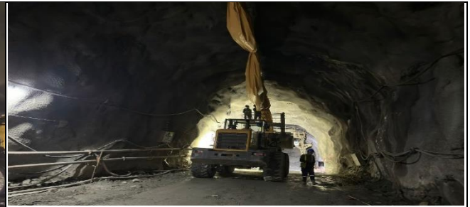
Extension of Ventilation duct
