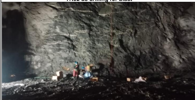
TRT02 US Charging.
