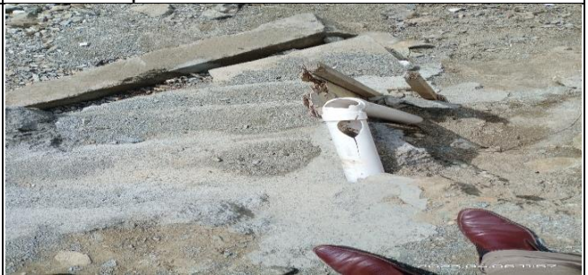
The broken internal water supply pipeline at Rv Uchar-01
