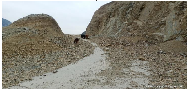
Loose material falling from the unprotected cuttings at internal access road of RV Uchar-01
