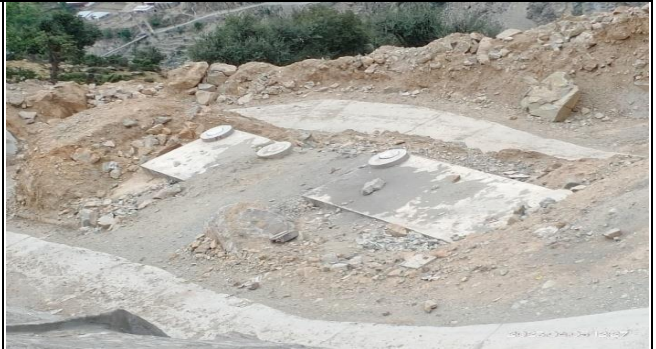
Septic and anaerobic tank at RV Nasirabad-02
