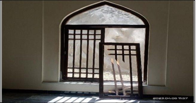
The broken window of Mosque at Rv Nasirabad-01
