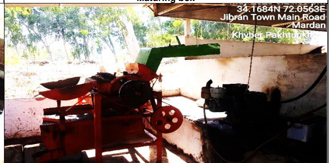
Shredder with generator
