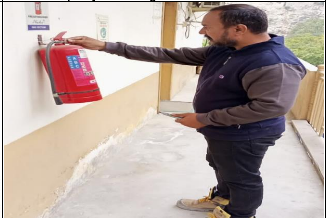
A view of Monthly inspection of portable fire extinguishers at DHC Office
