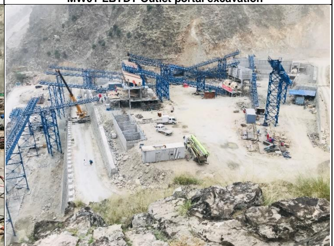
MW-01 & MW02_Uchar Crushing & Batching Plant at Thoki
