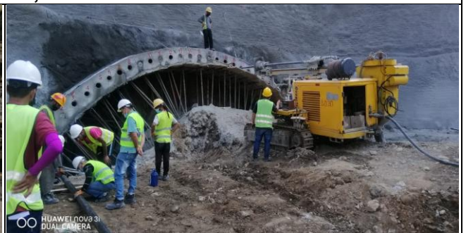
Drilling & installation of Canopy pipes at Inlet Portal of Logro A tunnel
