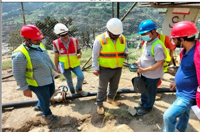
Verification of resistance measurement by DHC OHS at switchyard
