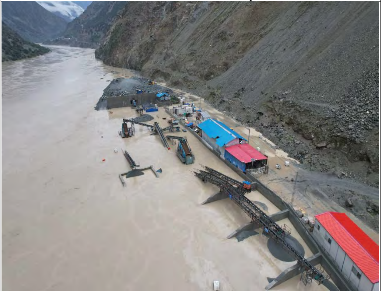
Submerged KKH and Uchaar Crushing plant
